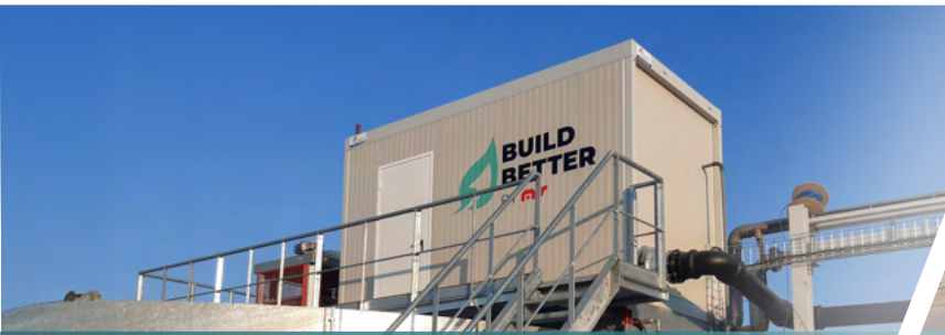
01 Control room, containing the flocculant preparation and dosing unit and the power cabinet
